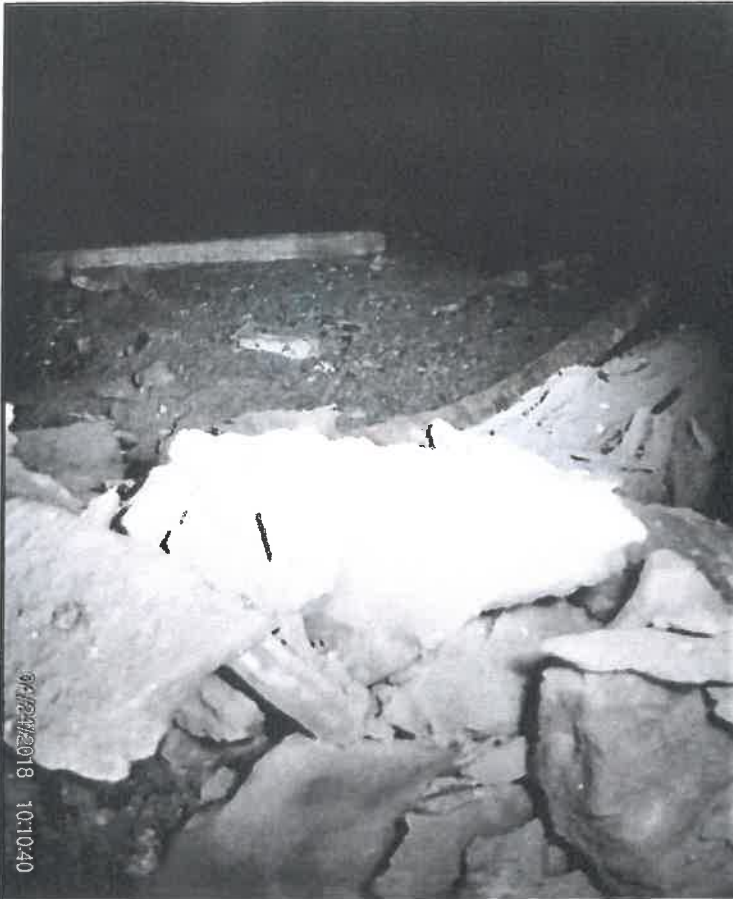
Floor of open mine shaft within boring B-8
