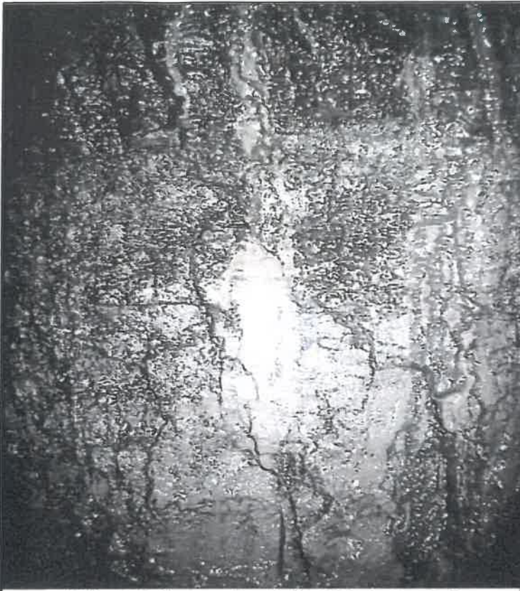
Side-wall of open mine shaft within boring B-7
