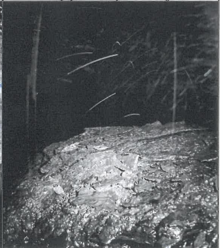
Floor of open mine shaft within boring B-11
